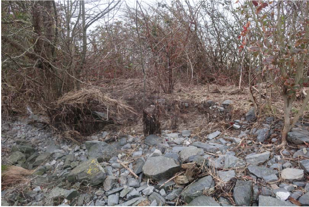
Another spill over location. Note upper level of dike has been eroded.
