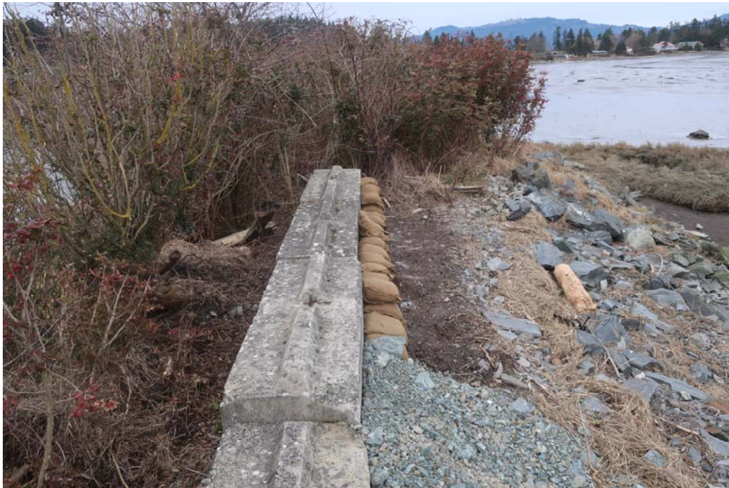
Combination concrete block, gravel and sandbag patch of eroded dike section
