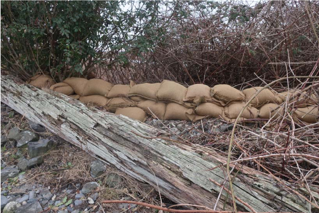
Sandbag patch at overflow location. Note driftwood log that was blocked by vegetation.
