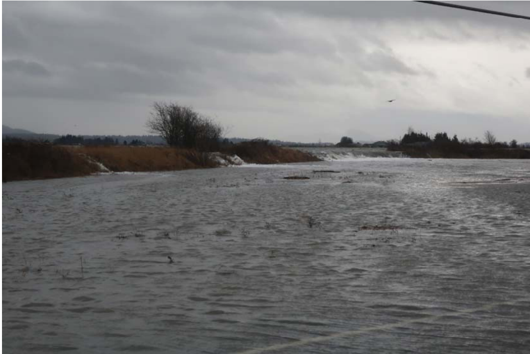
Note elevation difference between tide and flooded area and the erosion of the top of the dike
