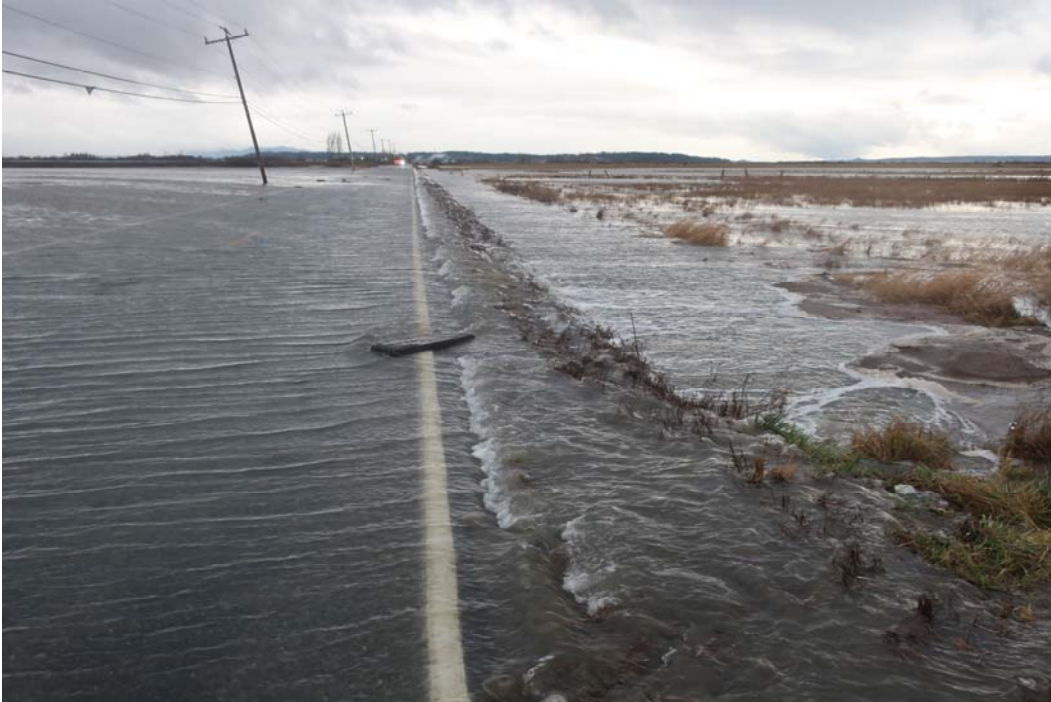
Water flowing over shoulder of road into deep ditch below the road. The ditch has been overtopped and saltwater is spreading across fields towards the west and south. The ditch drains to the north to Drainage District #5.
